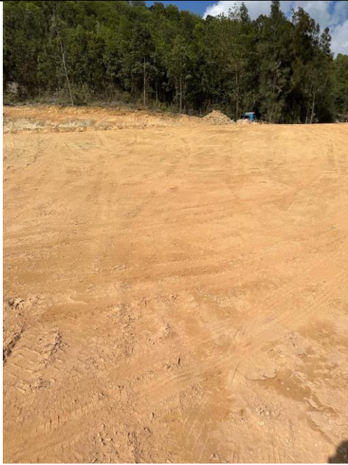
4. The work area in Portion A is dry and fugitive dust is observed.
