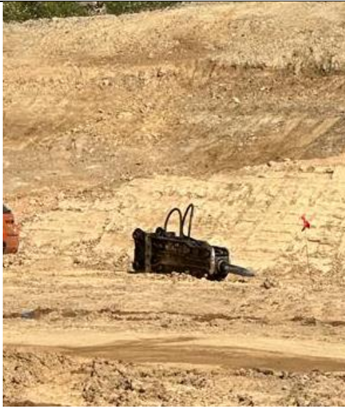
5. The plant equipment in SBA is placed on the ground without impervious sheets.
