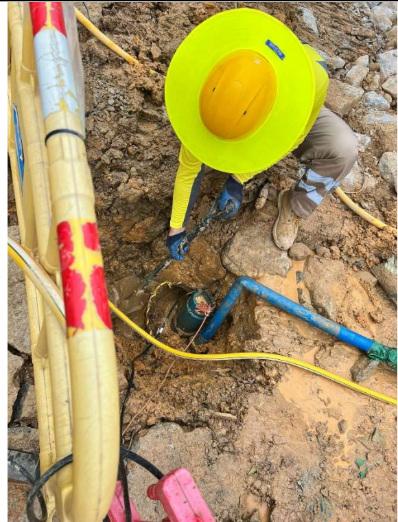
The sand and silt in the sump pit and the channel at the vehicle were removed.
