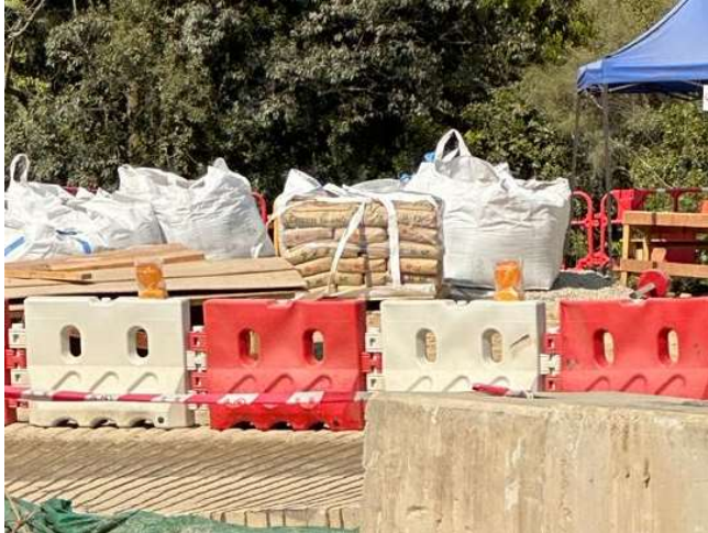
3. More than 20 bags of cement were not covered entirely by impervious sheets in SBA.
